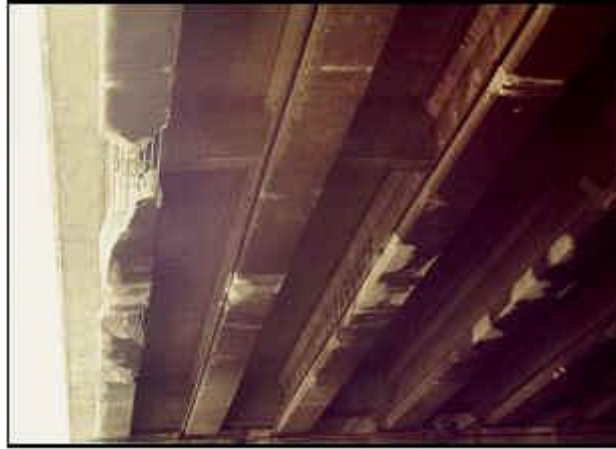
Figure 4.1 Collision Impact on Exterior Girder
